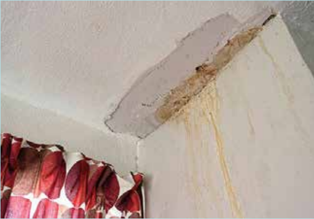
Penetrating damp (above)
