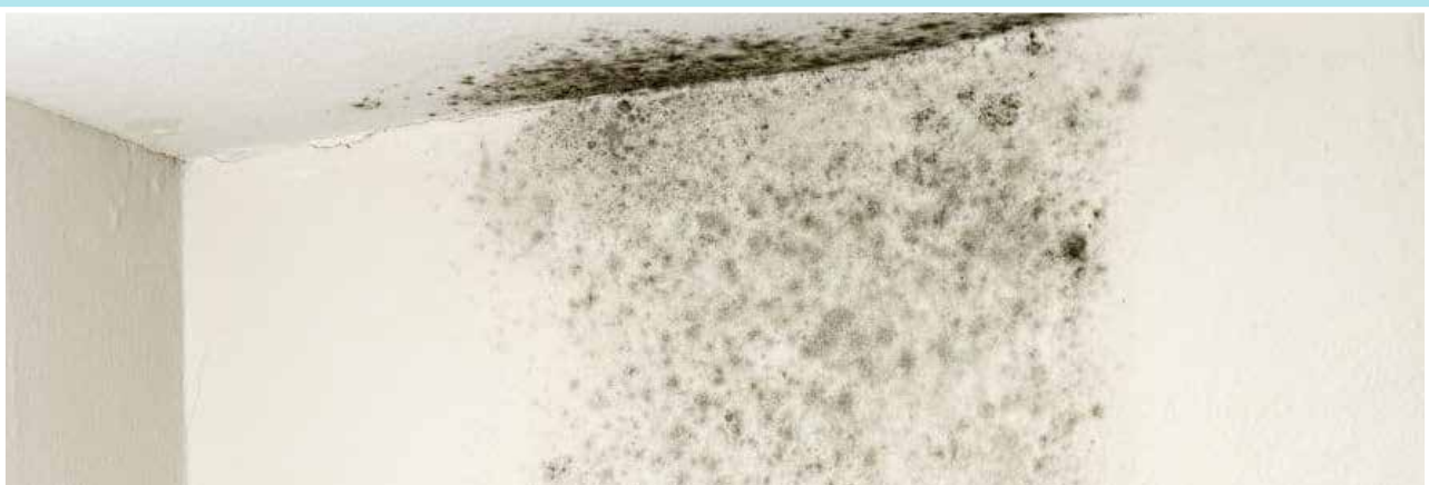
Mould caused by penetrating damp (above)
