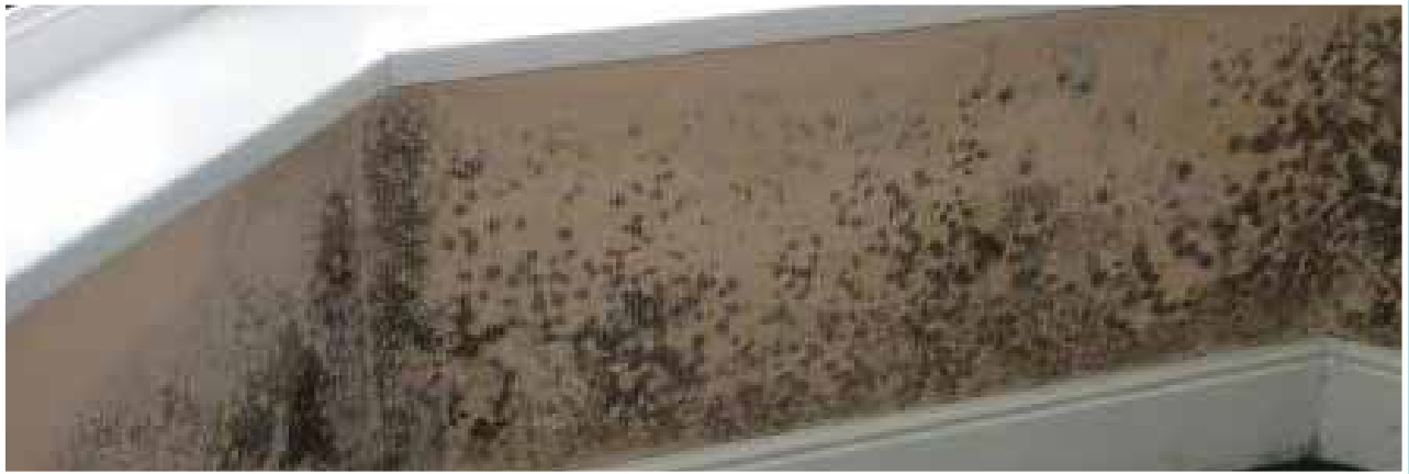
Damp caused by condensation (above)
