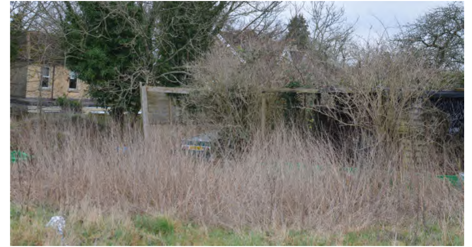
3. Existing dilapidated shed located on the eastern boundary of the Site, identified as a potential bat roost opportunity location.
