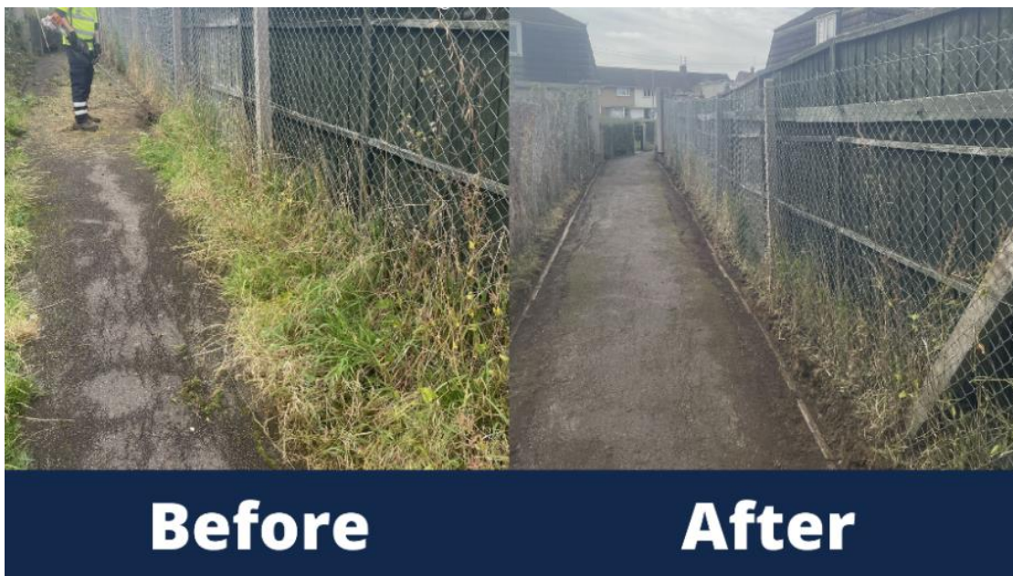
Alleyway cleared of weeds from Tenby Road to Coronation Avenue in Keynsham
