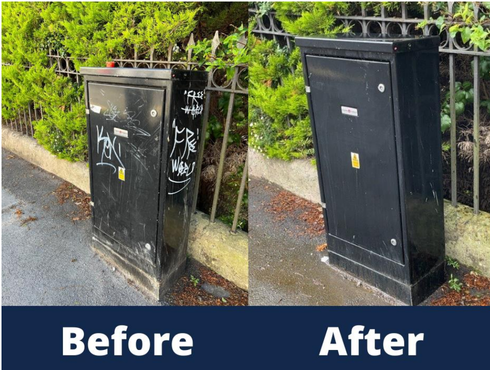
Graffiti removed from a utility cabinet on Raby Place in Bathwick
