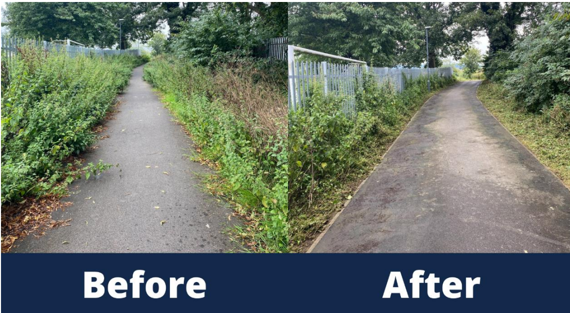
Vegetation trimmed on Norton Hill to support pathway clearance in Midsomer Norton
