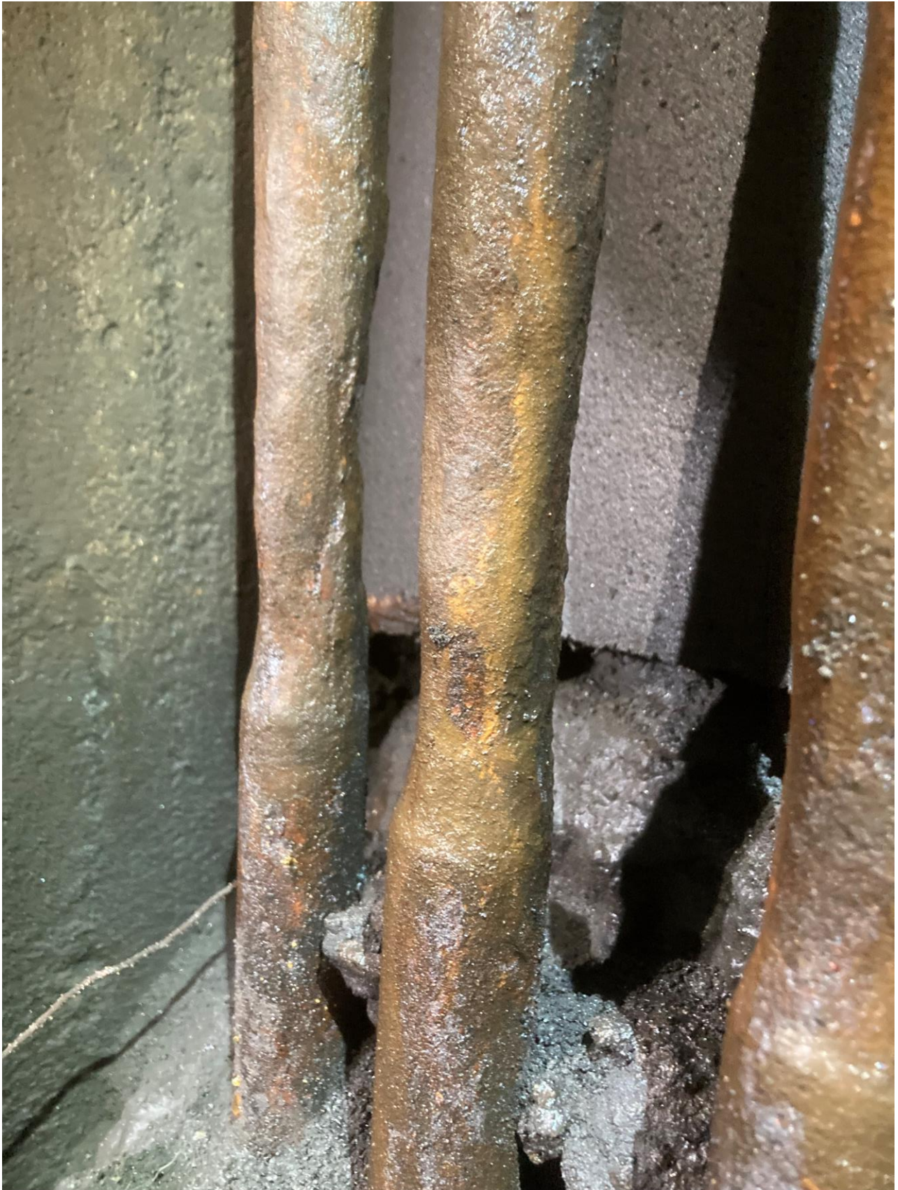
Figure 3 - Close up photograph of hanger bars to the north end of Truss No.4.
