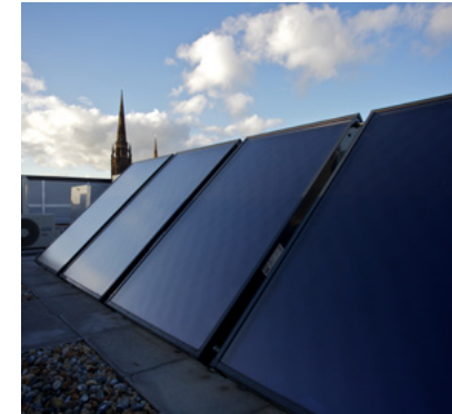
Solar photovoltaic panels for electricity generation
