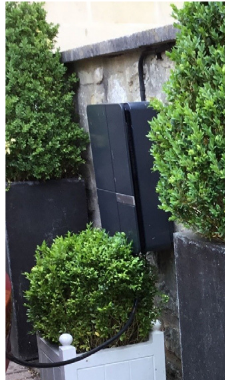
A discreetly-located Electric vehicle charging point within a residential curtilage in Bath.
