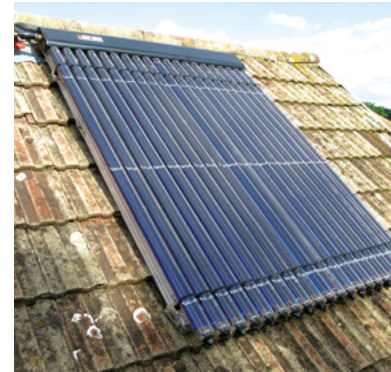
Solar thermal panels for hot water
