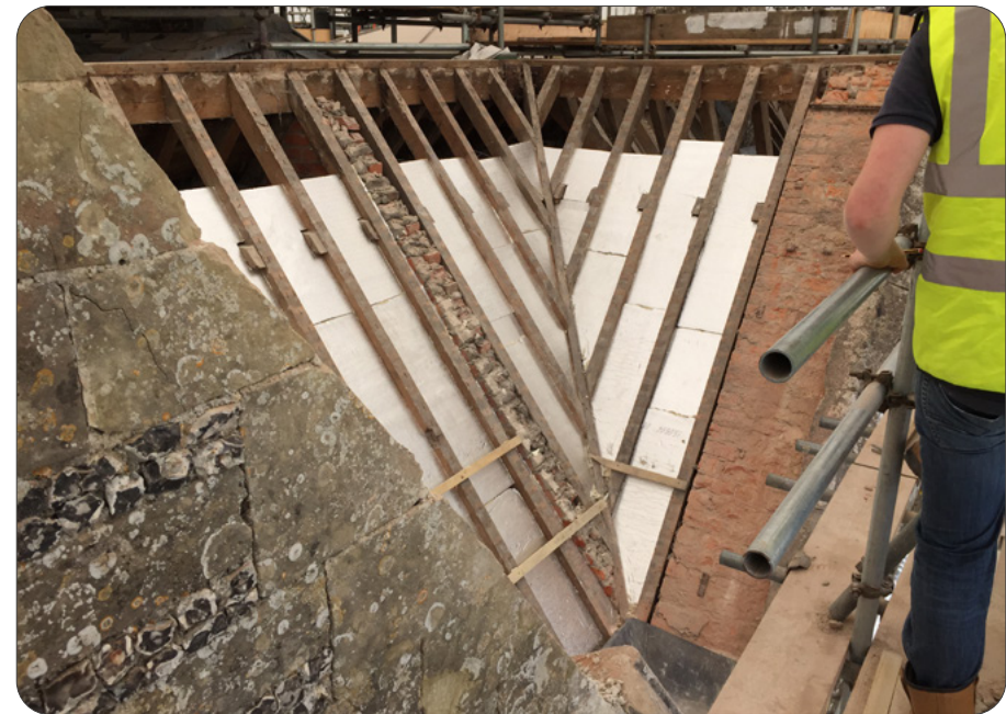
Each eaves detail needs careful thought once insulation is added. Often bespoke solutions have to be devised to achieve effective improvement
