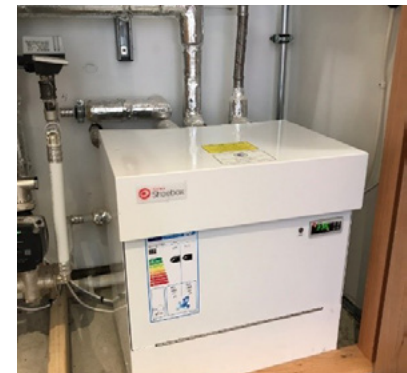
Ground source heat pump
