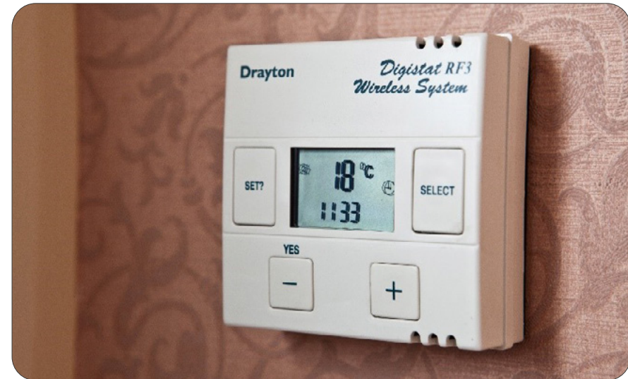
Adjustable heating control. Photo copyright: The Centre for Sustainable Energy
