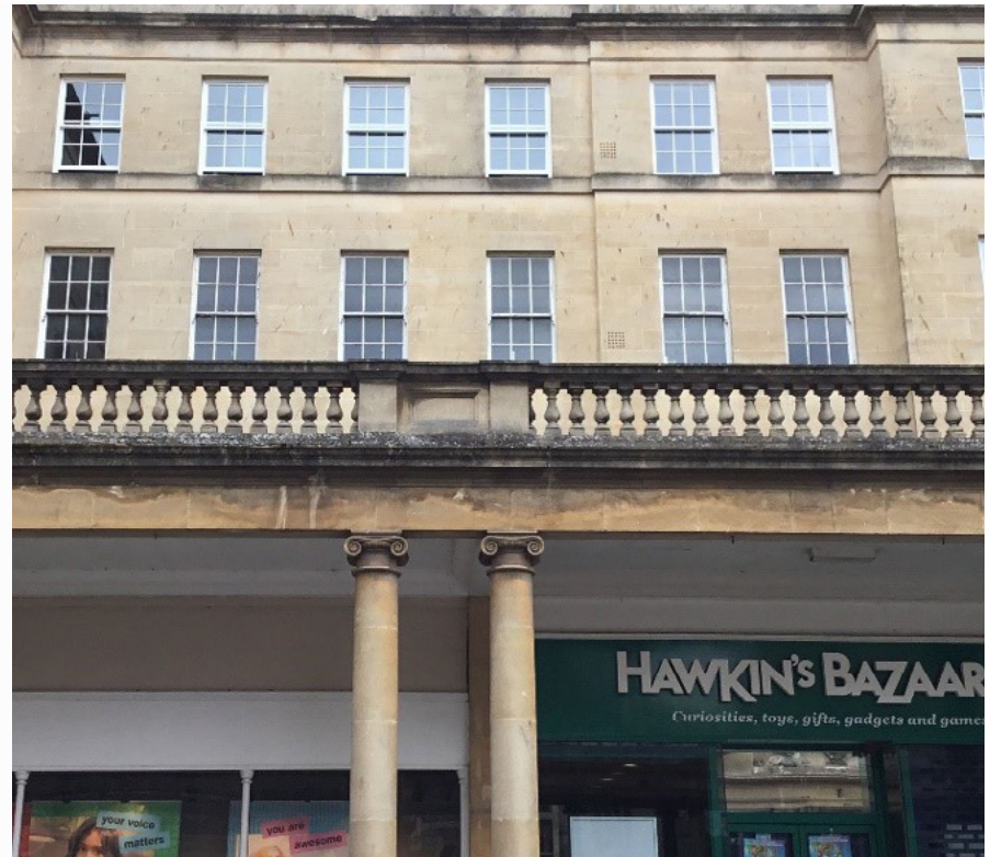
Replacement slimline (12mm) double-glazed sash windows alongside existing original single-glazed windows in Arlington House, Stall Street, Bath.
