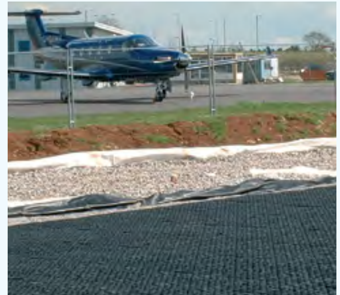
Bristol Airport Car Park permeable paving
