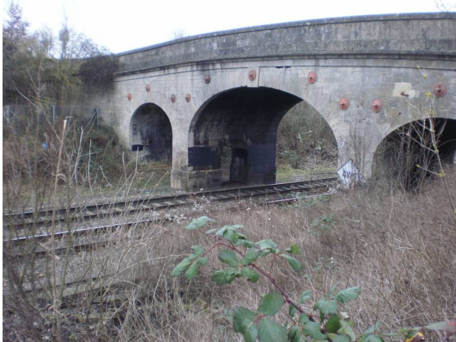
Photo 3.3 Mill Lane bridge west elevation photographed from George Inn PH car park
